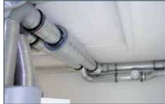
Air duct system in an office complex
