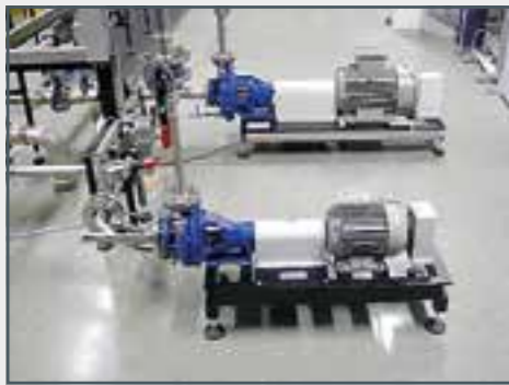
HM 124 pump station
