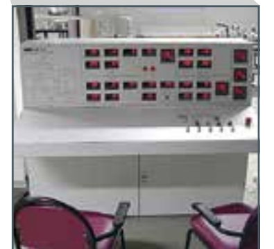
The industrial scale control console ensures a clear and convenient operation.
