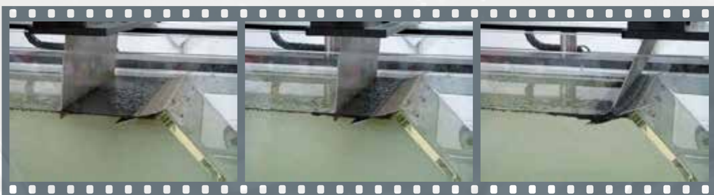
The electrically driven scraper clears the float from the surface of the water.
