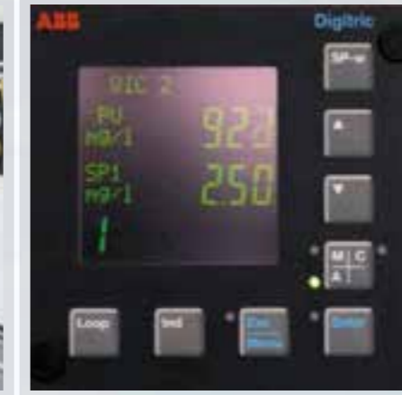
Digital industrial controller
