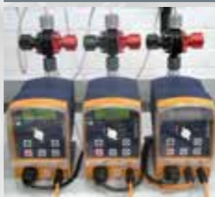
Precise addition of chemicals by use of industrial metering pumps
