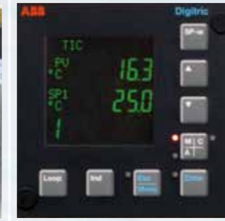
Digital industrial controller
