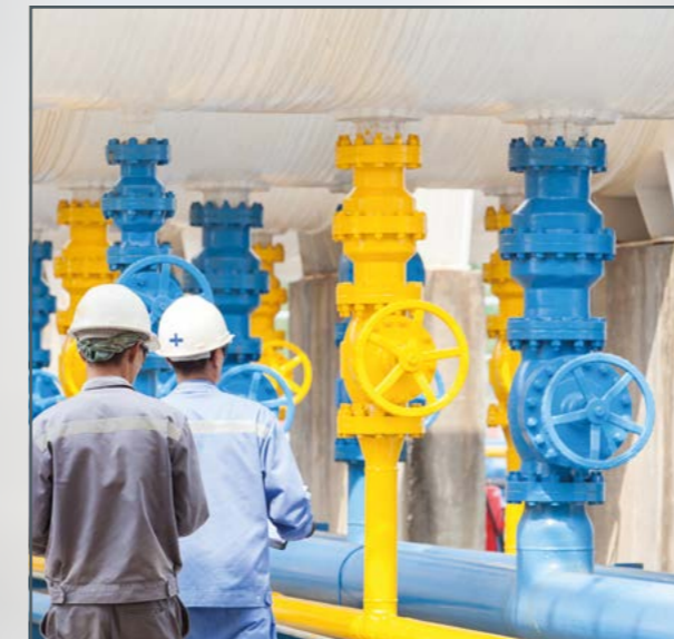
Valves and fittings of a large-scale distribution station
