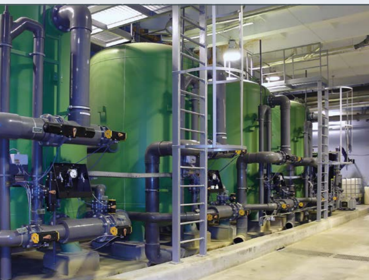
Continuous-flow adsorber in a water treatment plant
