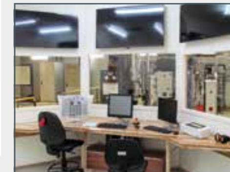
Module D control station
